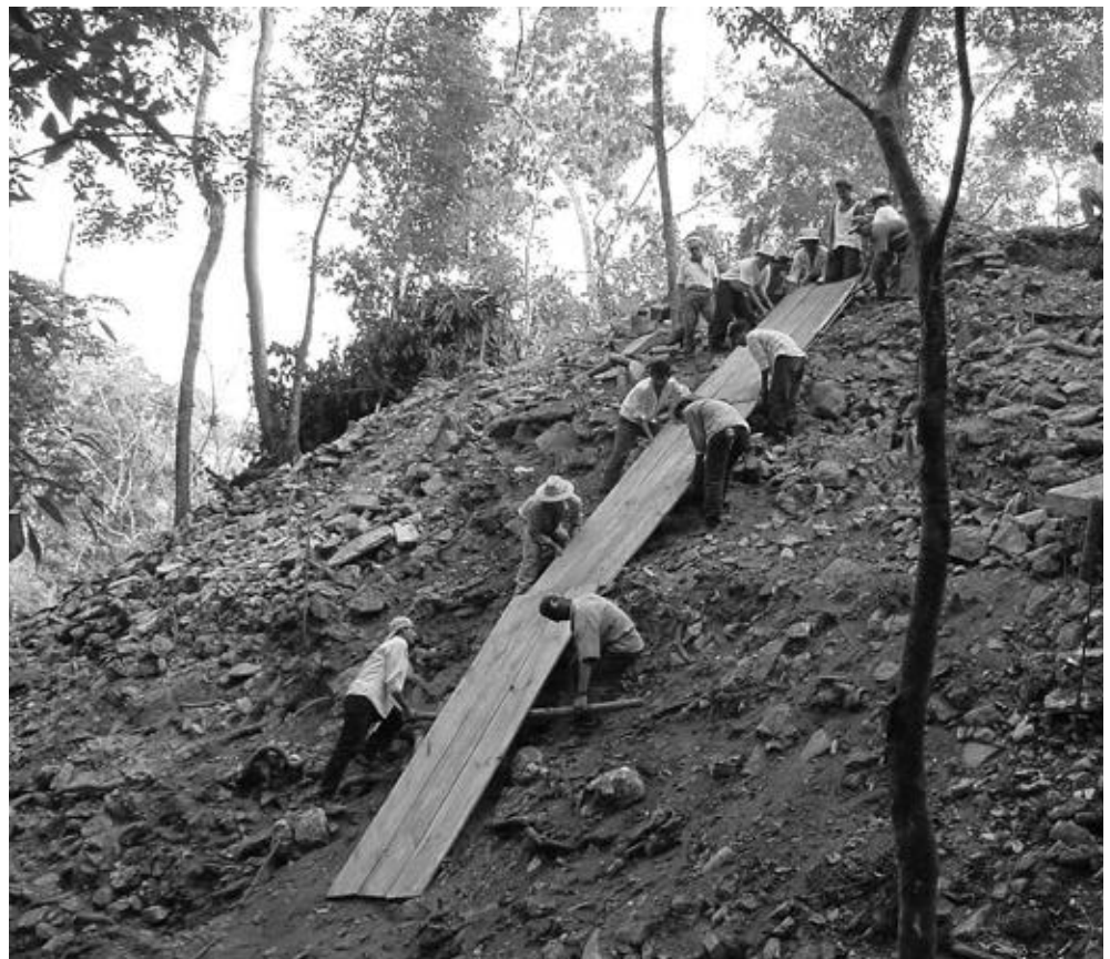
Photo showing Structure XIX with a wooden ramp to remove rubble and excavation debris from the walls (on the southern side of the structure)
