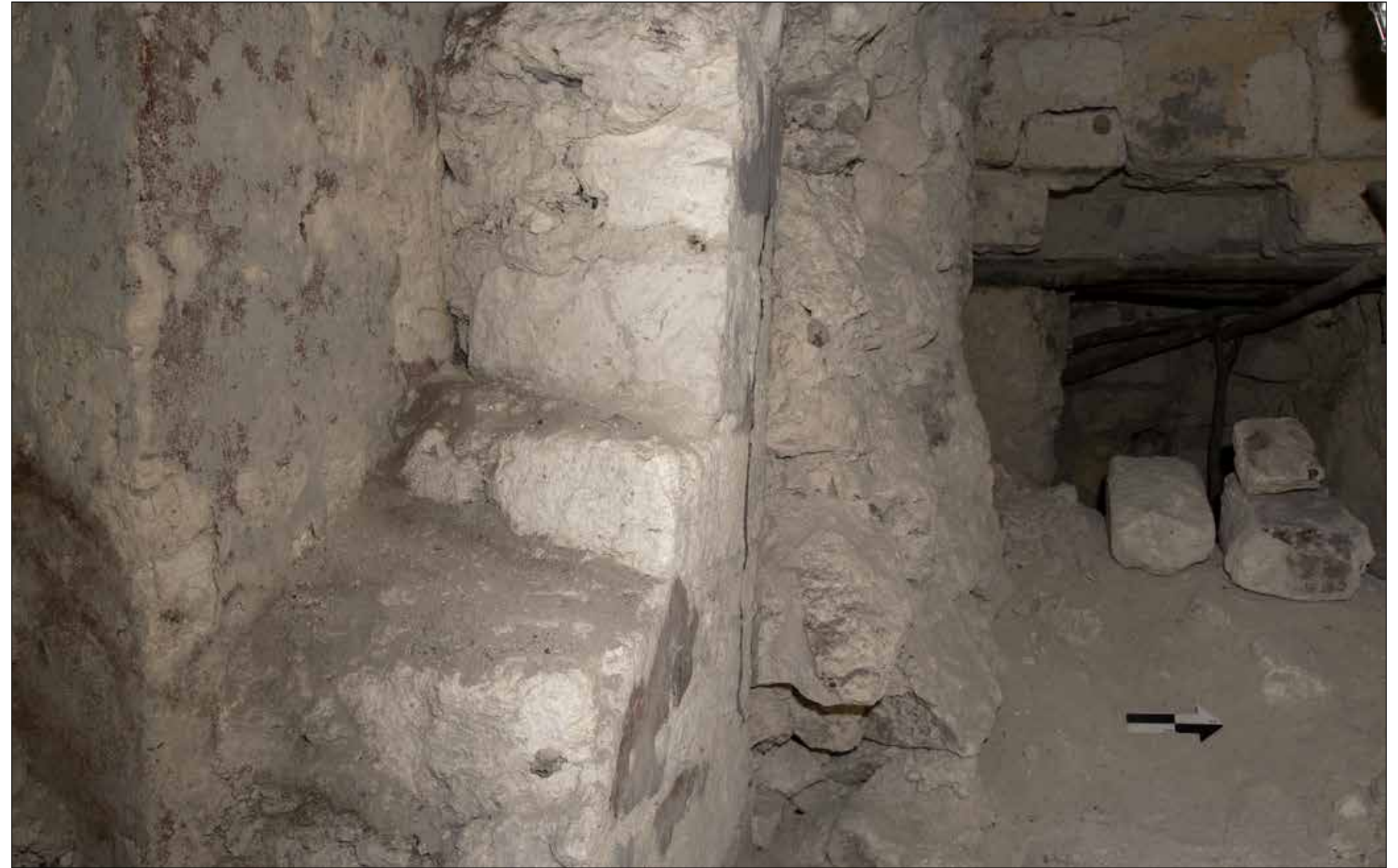
Figure 2.30. Front chamber of Temple of the Night Sun, reinforced by thickening the door jamb of its middle wall to combat structural failures. Photo: Arturo Godoy.
